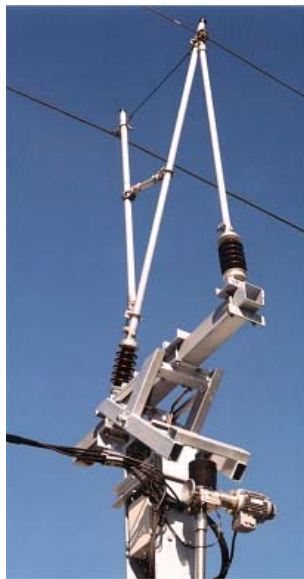
Figure 11.3: The mast in the up position with the tilted contact wire
